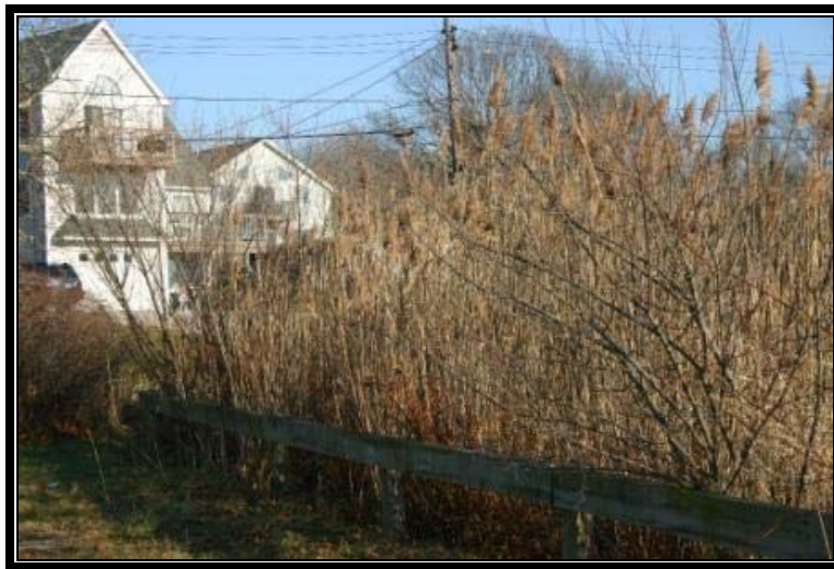
Whoa! This swale is so full of sediment and invasive plants it no longer treats stormwater runoff.
