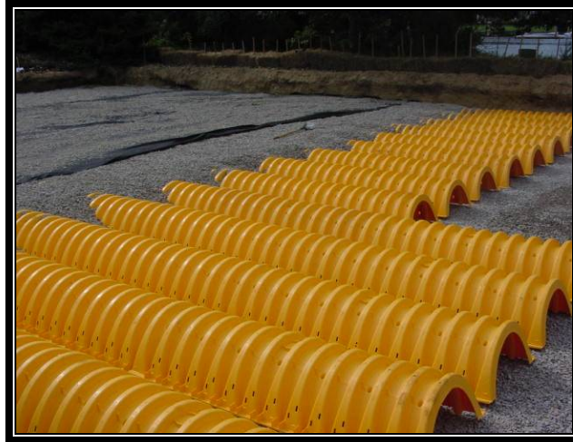
The Town of Narragansett installed an infiltration system under a parking lot to treat stormwater from a storm drain, before it enters Narrow River.
