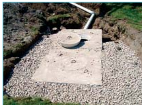
Installed infiltration chamber
